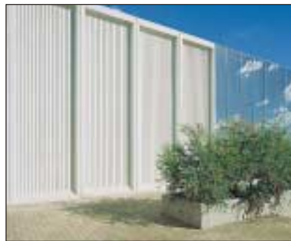
Top quality Class 2 off-form finish in industrial building representative of best industry practice
