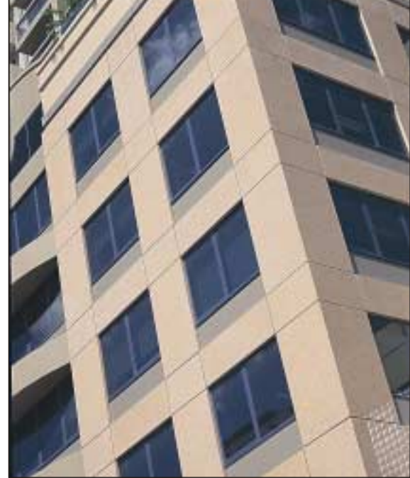
High-rise office building clad with high-quality polished facade panels providing Class 2 finish – the best the precast industry can produce
