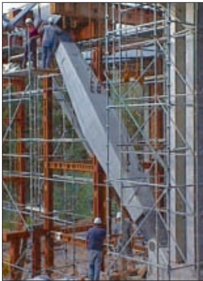
Erection of precast spandrel tension tie (note temporary stability support for wall)
