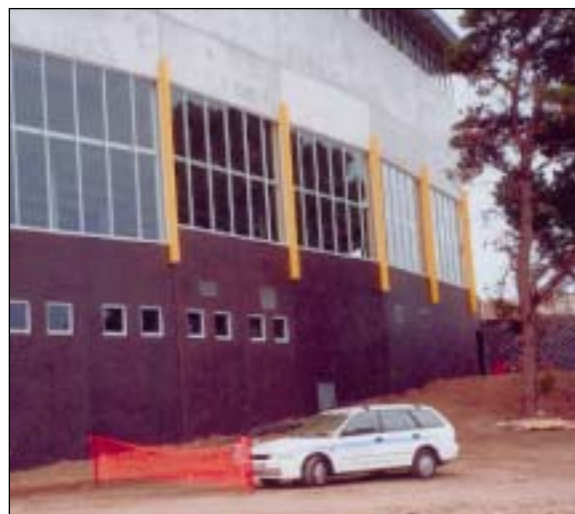
Rear view of Southern Stand showing 6.5 m height coloured precast wall panels
