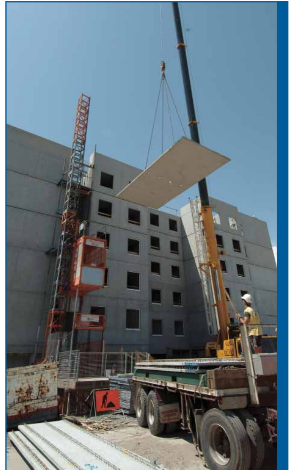
More than 3300m 2 of precast flooring were supplied for the Mascot Hotel.
