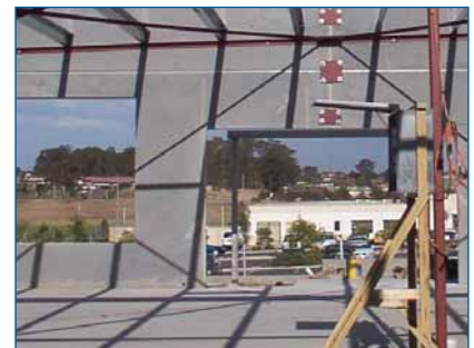
Precast walls in the new KFC Richmond include architectural recesses, penetrations for mechanical equipment, connection points for structural steel and connection points for adjoining panels.
