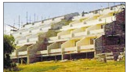
7.5-m HC planks spanning two occupancies, utilising plank properties. Note use of HC plank as balcony parapet wall
