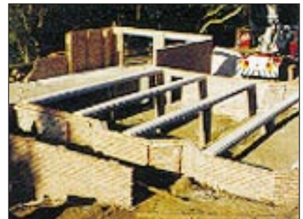
Resdek beams on engaged piers with intermediate piers as required by span and spacing
